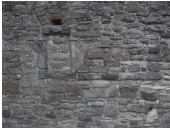
Figure 30: Area around a blocked-up window.
